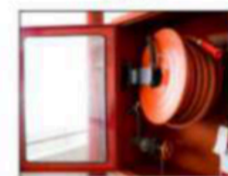
Fire fighting System
