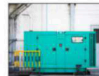
Power Back-up for Common Area
